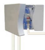
Mains water top-up panel
